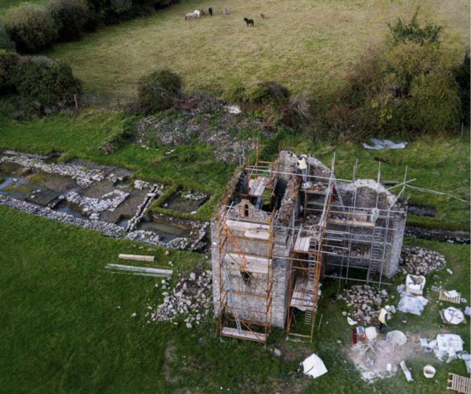
Aerial view of the Beabec service tower during conservation works with the outline of the great barn beside it (photo: National Monuments Service)
